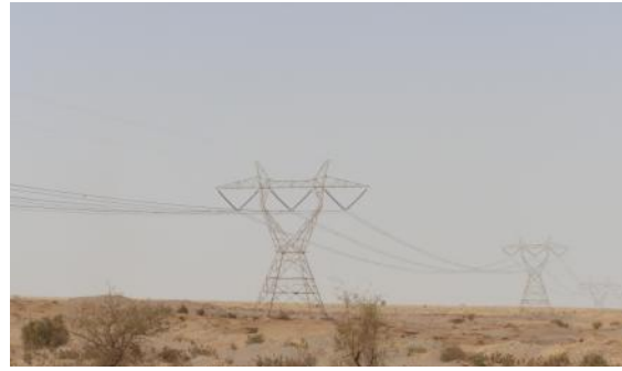
2 - Existing transmission line
